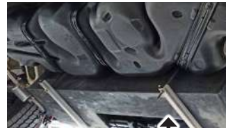
Gray Water Tank
