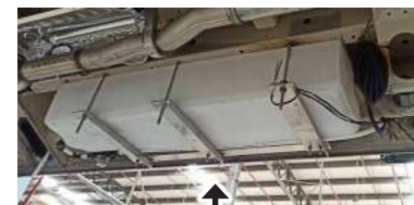
Fresh Water Tank
