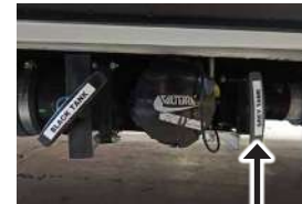
Gray Water Tank Valve
